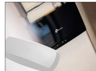
Extern antenn router
